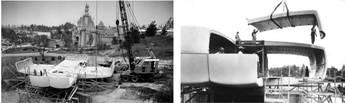
Construction images of The Monsanto House of the Future under construction in 1957 in Disneyland, California
